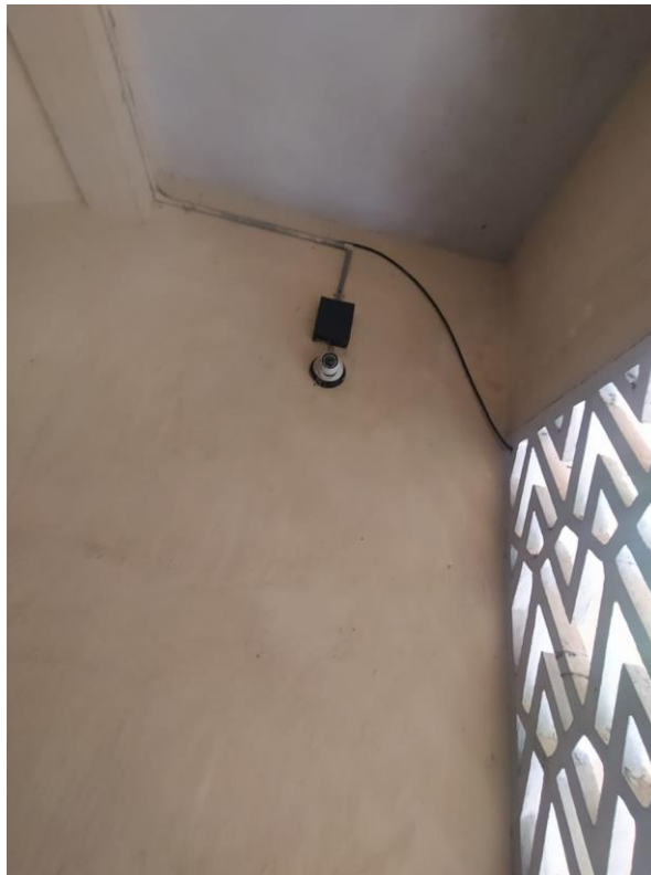
Photo view of CCTV (Administrative Block)
