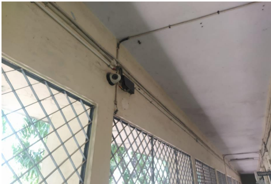
Photo view of CCTV (Computer Block)
