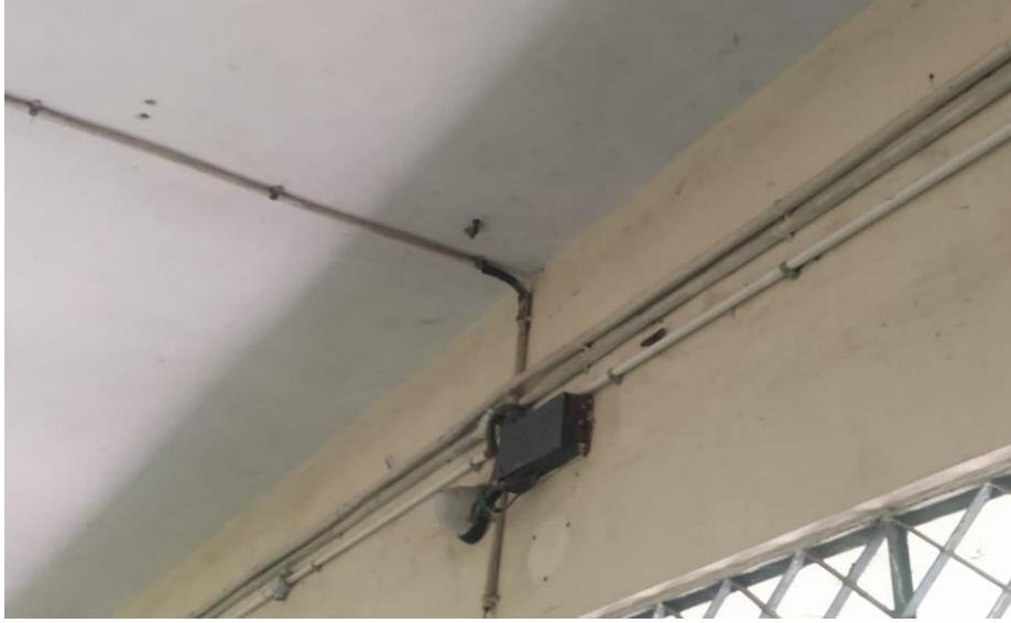
Photo view of CCTV (Computer Block)
